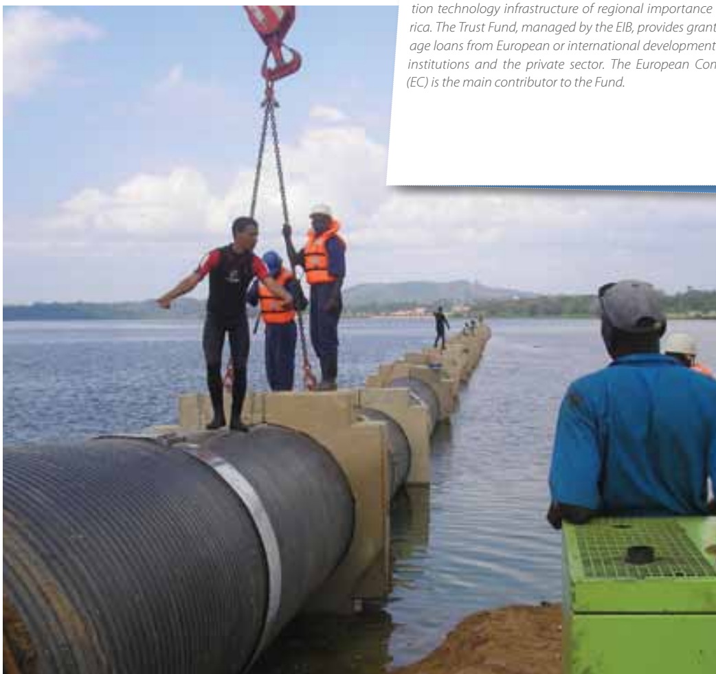
Gaba offshore pipeline, Kampala, Uganda
