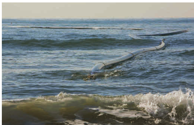
Submarine power cable, Italy
